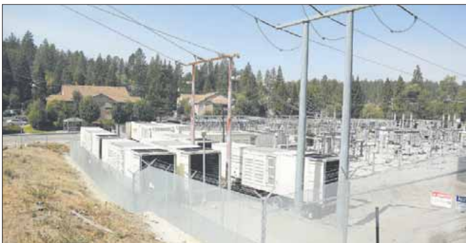
A temporary power generation station set up at PG&E's Brunswick Substation uses diesel-powered generators the size of 10 shipping containers. Power from the Brunswick and downtown Grass Valley substations are keeping the population cores of Grass Valley and Nevada City energized with power during the Public Safety Power Shut-off.
